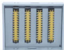
Junction Box 4 TP
