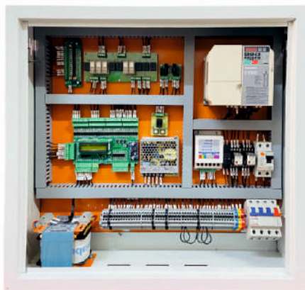
Elevator Geared Controller
